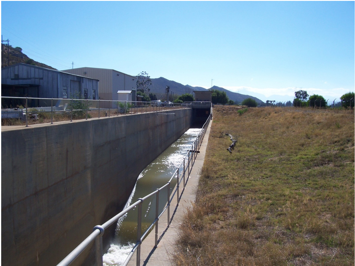
Figure 3: View of the pump station from the wave suppressor towards the tunnel
