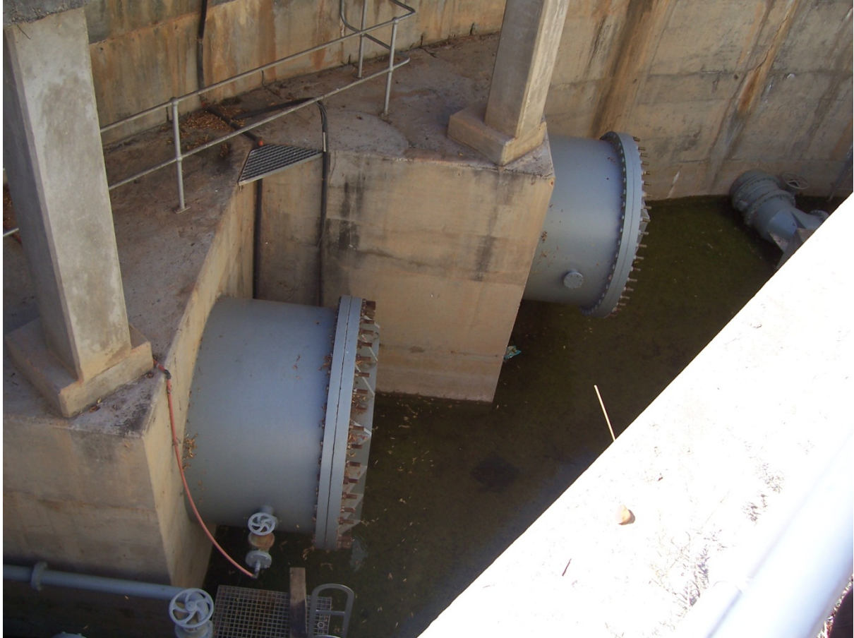
Figure 2: Blanked off pipes that can link pumping stations 2 and 3 with the tunnel
