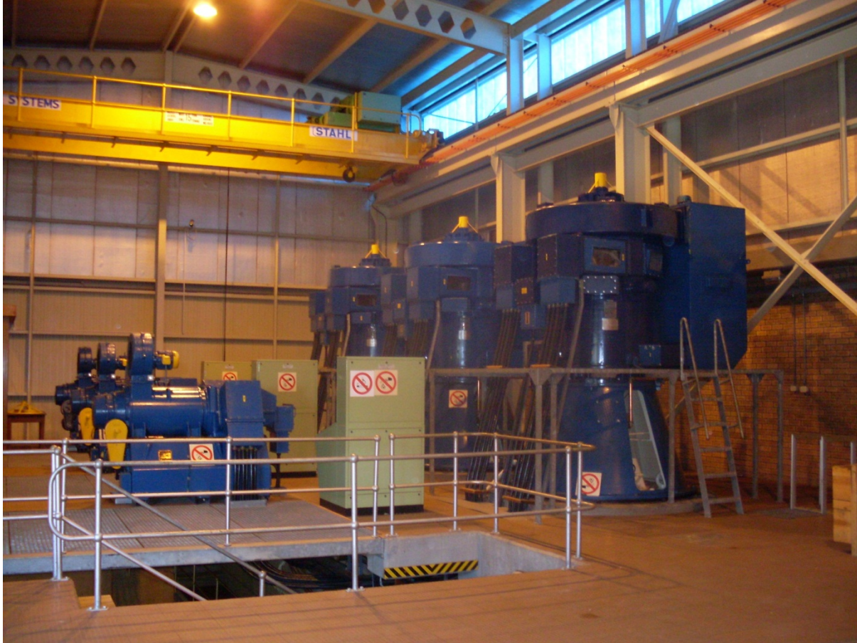
Figure 4: The interior of Papenkuils Pump Station showing the currently installed vertical turbine pumps
